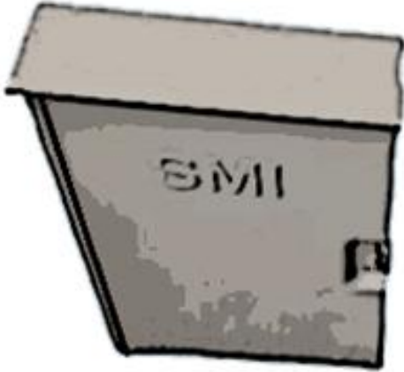
Weatherproof Cap Installed (Outdoor Rating)
